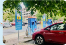
Top-of-bay chargers, The Range car park
